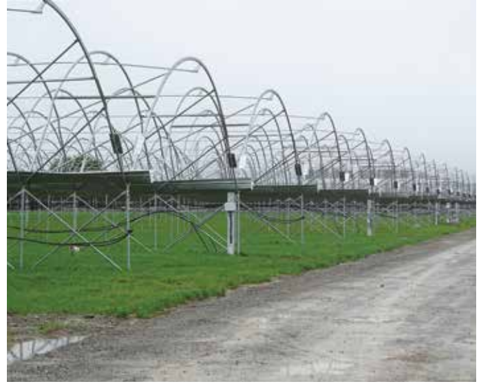
Construction of the strawberry development will be completed in time for planting
