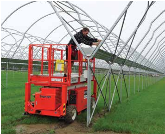
JS Ewers employee Kent Elford works on the construction of the 4ha development
