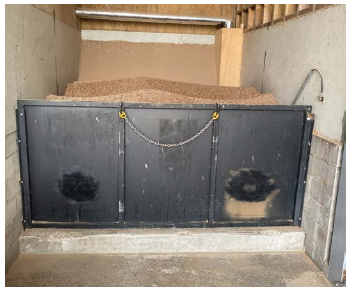
The covered area for storing the wood pellets is big enough for them to be tip loaded to drop into the feed system. Coal to wood pellet use is close to 1:1 so huge storage bunkers are not necessary
