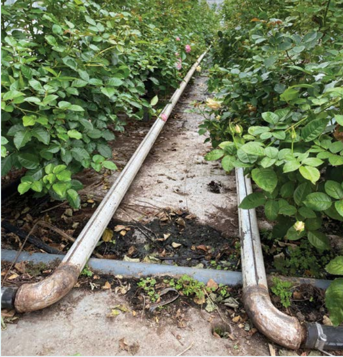
Pipes bring heat into the greenhouses
