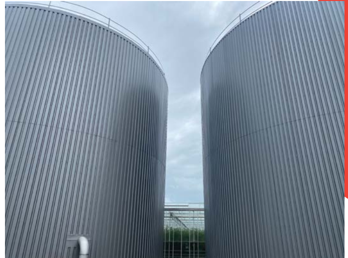
The newly installed buffer tank allows the storage of hot water with minimal heat loss
