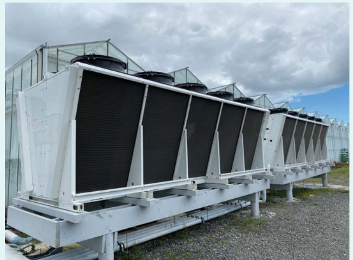
Airside evaporators at Van Lier Nurseries
