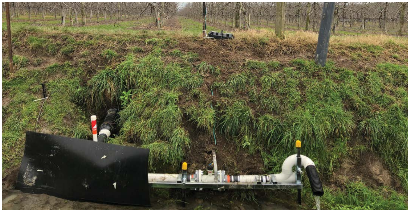
Installed in drain sampling equipment
