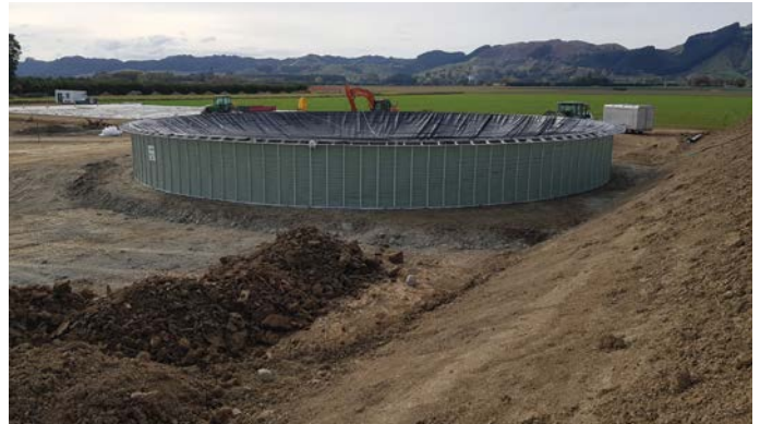
A large KlipTank installation in New Zealand. Photo courtesy of KlipTank
