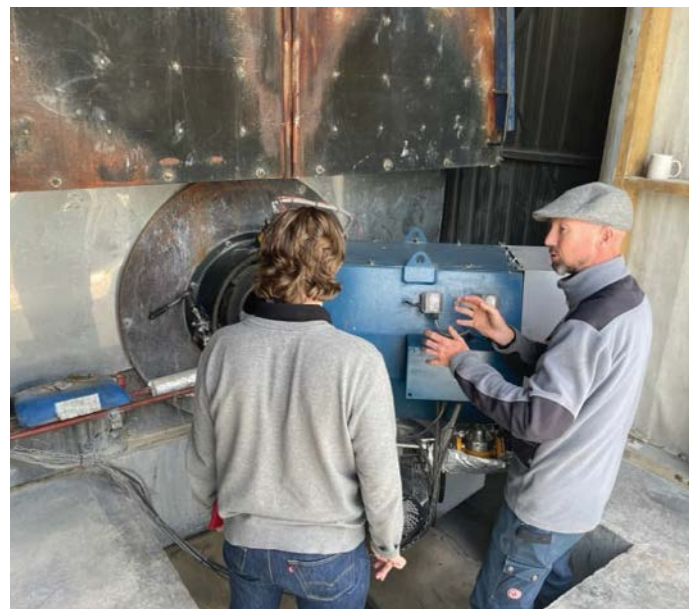
Ellery Peters and Robert Lindsay look at Jade Garden's glasshouse boiler to assess its potential for biomass conversion
