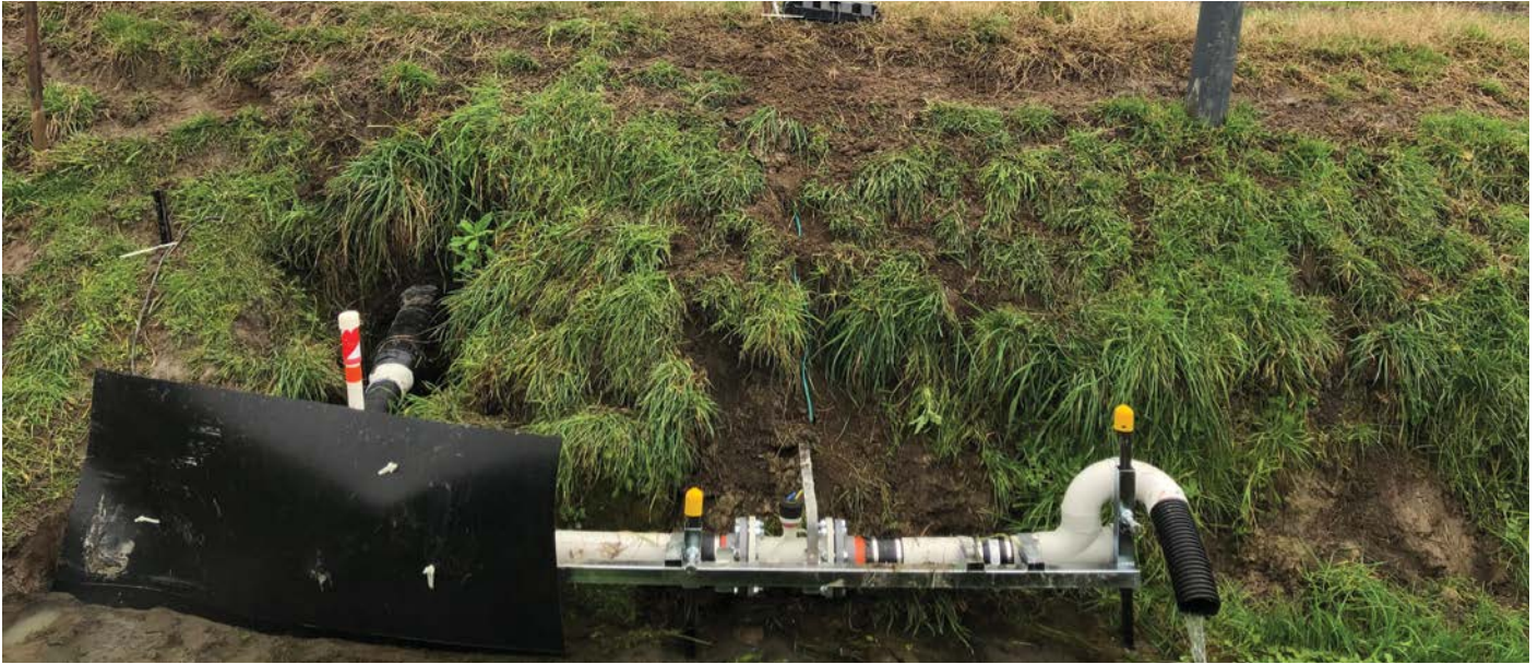
Installed in drain sampling equipment
