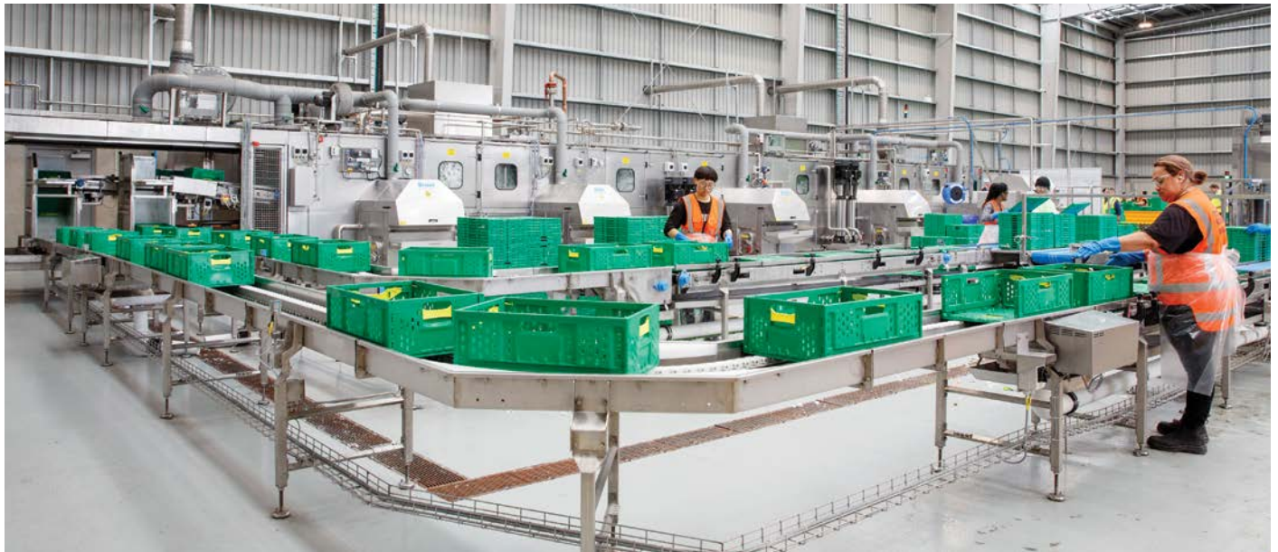
A new facility in East Tamaki will increase crate washing and drying capacity by 250 percent
