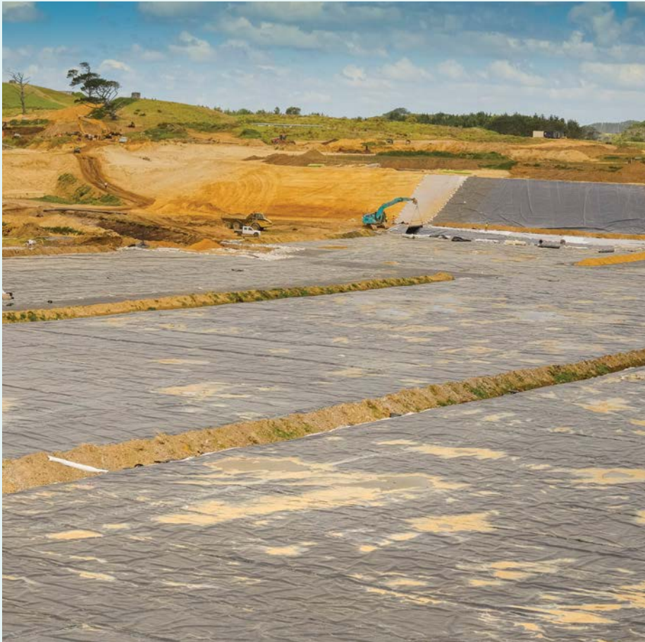
Once completed Te Waihekeora reservoir at Redhill on the Northern Pouto peninsula will hold sufficient water to support around 1100ha of new horticultural development
