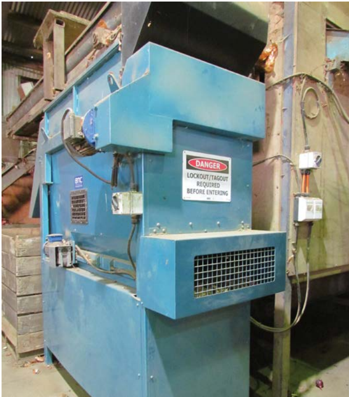
The onion scroll topper was modified after the accident and signage improved
