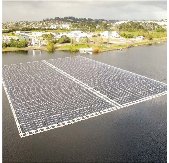
Believed to be the only floating solar array in operation in New Zealand, Watercare's Rosedale Wastewater Treatment Plant in Albany is a great example of using a pond's surface area to generate power for on-farm use and / or export to the grid, which can partly offset the lost production from the pond area. Photo courtesy of Watercare
