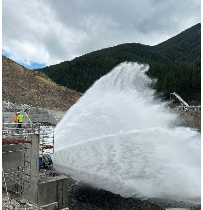
The first valve opened in March to release water. Photo courtesy of Waimea Water
