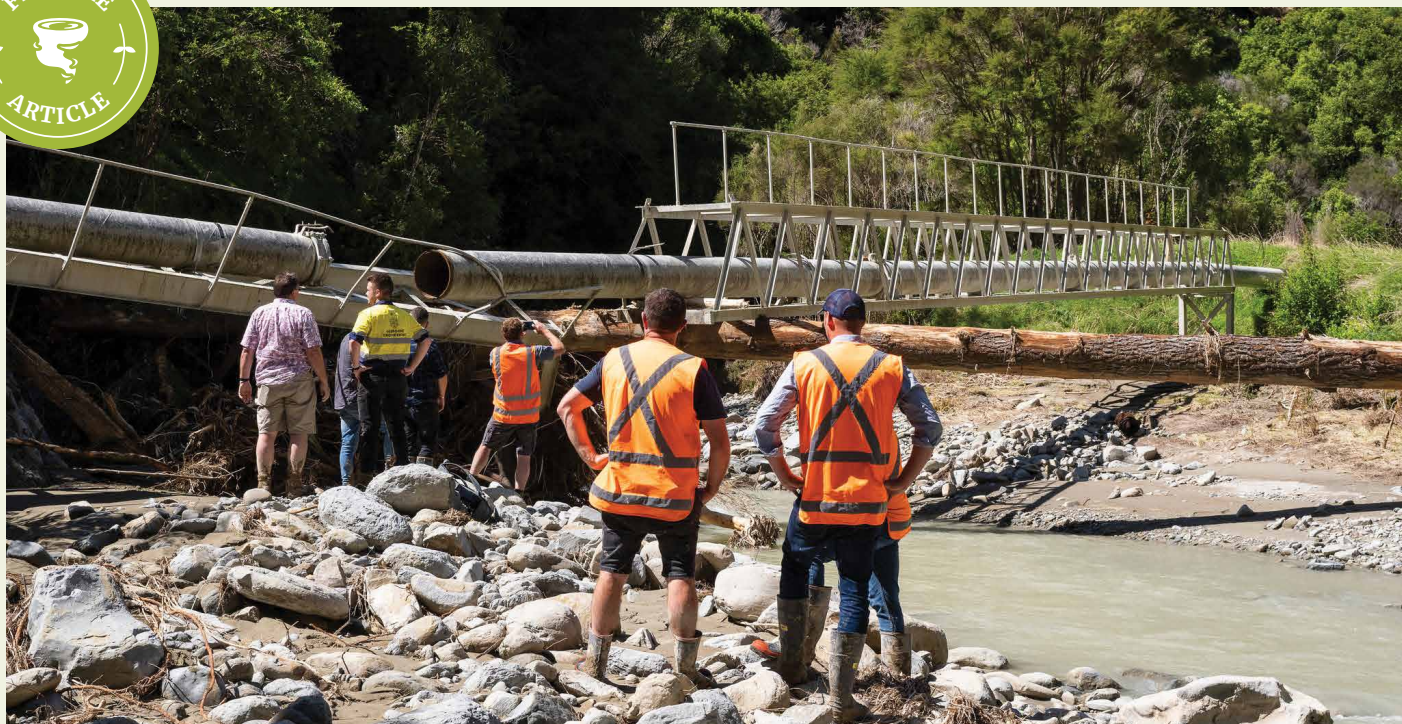
The cyclone caused infrastructure damage which heavily disrupted water supply in the Tairāwhiti area
