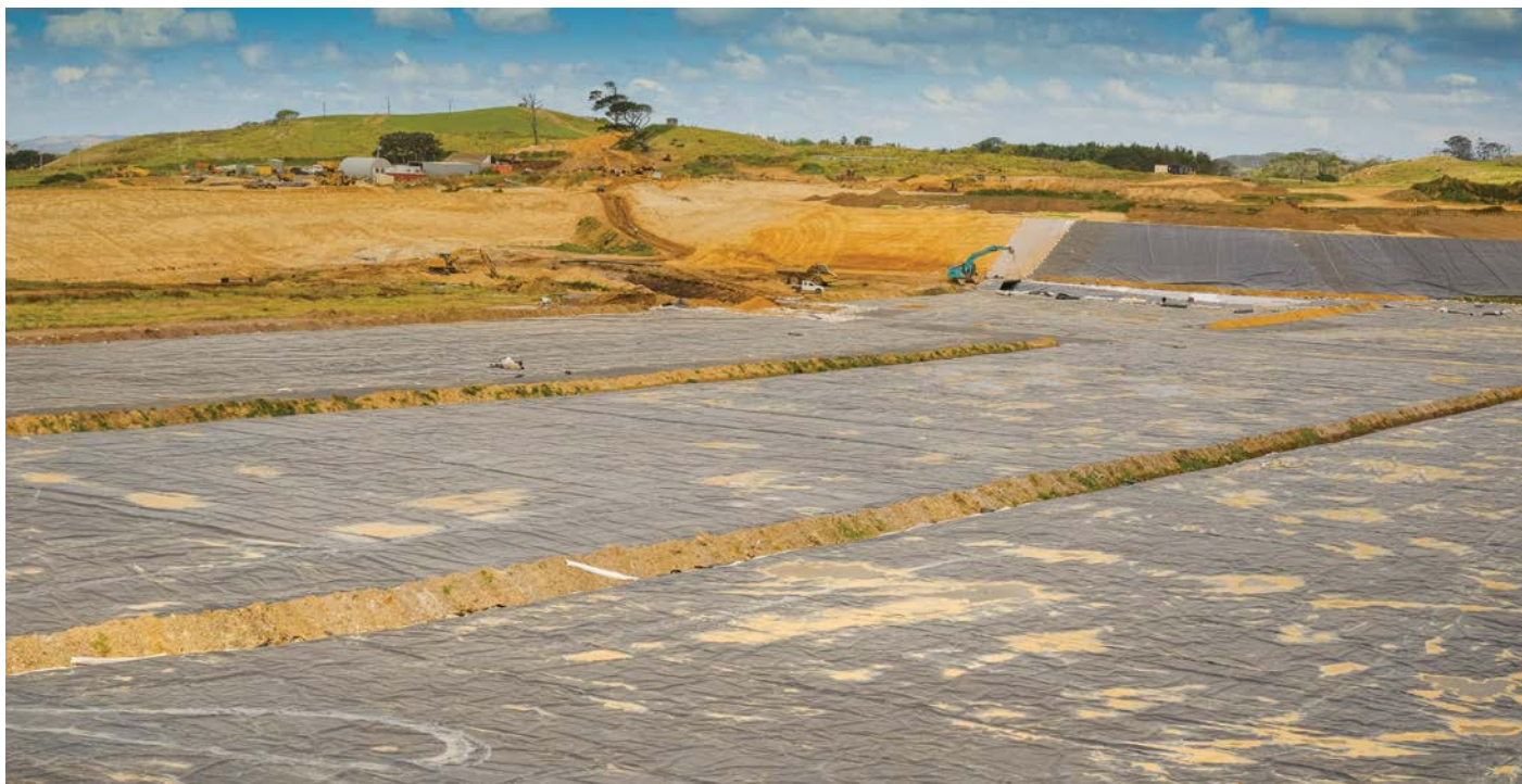
Once completed Te Waihekeora reservoir at Redhill on the Northern Pouto peninsula will hold sufficient water to support around 1100ha of new horticultural development
