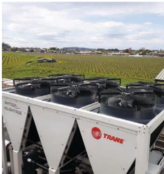
Trane, European made air-cooled chiller
